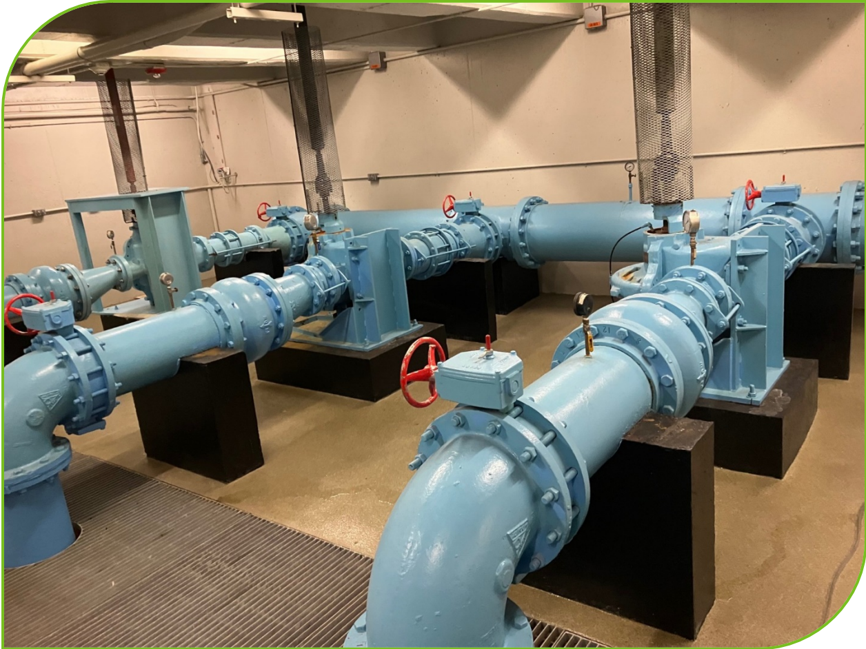
Water Station Interior
