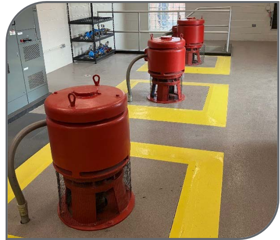
Water Station Pumps (Will receive generators in FY 25/26)
