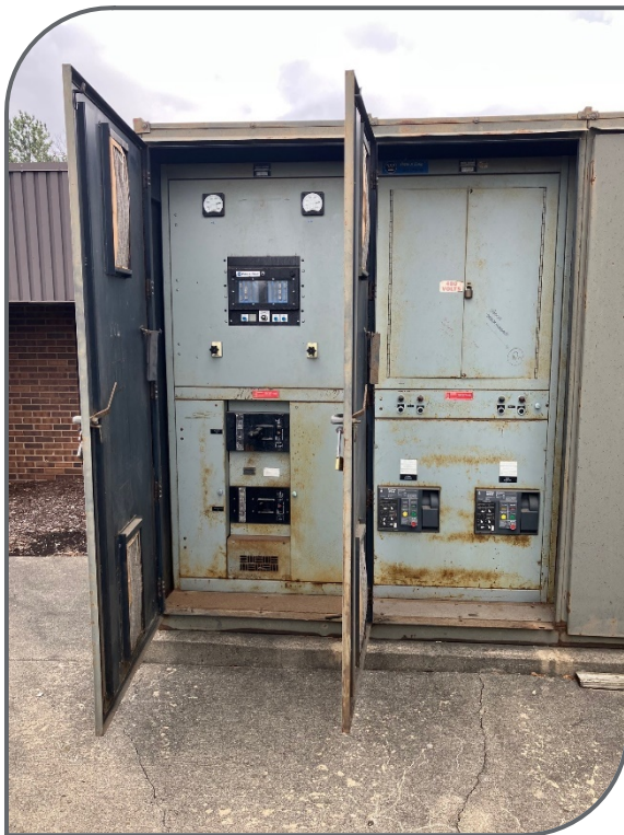
Current ATS condition of Stations 20 & 21
